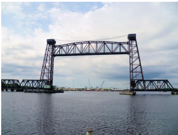
One of the railroad lift bridges on the ICW in Norfolk, VA
