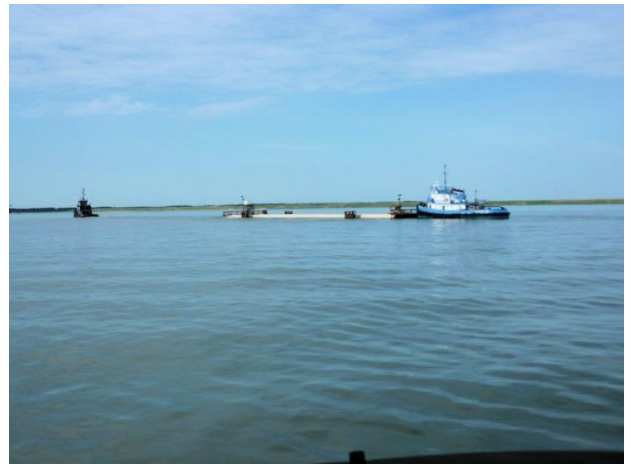
A section of road tunnel made in Baltimore and towed to Norfolk, VA
